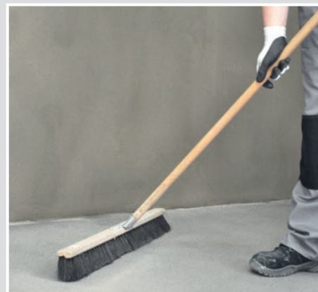
When the epoxy has dried accordingly, broom sweep and vacuum the surface removing any loose sand.
