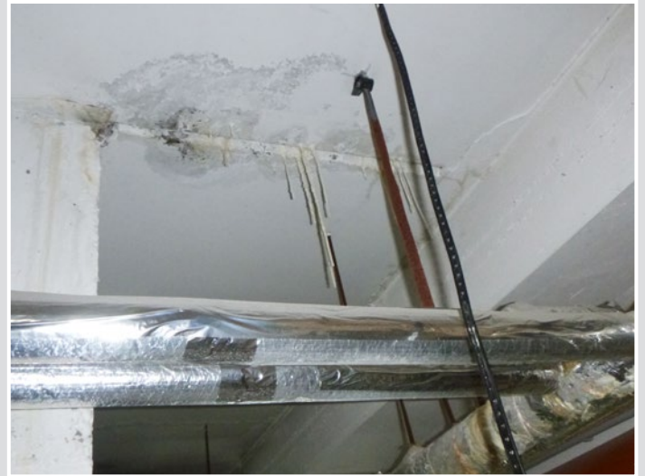
'Communicating tubes' without the sealing of the capillaries and water proofing tapes resulting in failures from penetrating moisture to the pool surroundings and/or the lower rooms.
