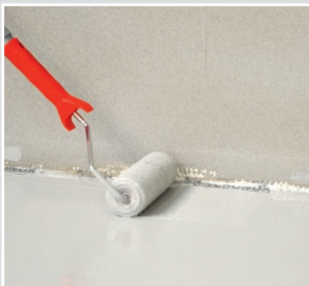
Within 12 - 24 hrs apply the coloured coat of SCHÖNOX EA PUR using a suitable roller.
